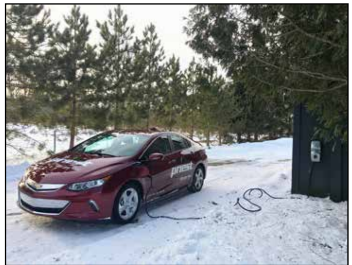
Priest Construction's Chevy Volt plugged into the charge station they recently installed at the author's home. Priest Construction has also installed fast charge stations at several malls around Montreal.
